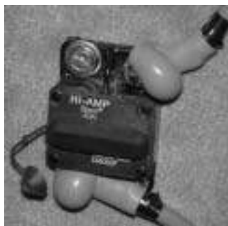
Figure 4-2. Main Circuit Breaker
