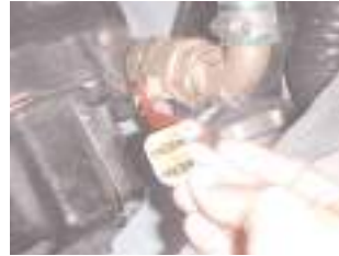
Engine Cooling Water Intake Shut-Off Valve
