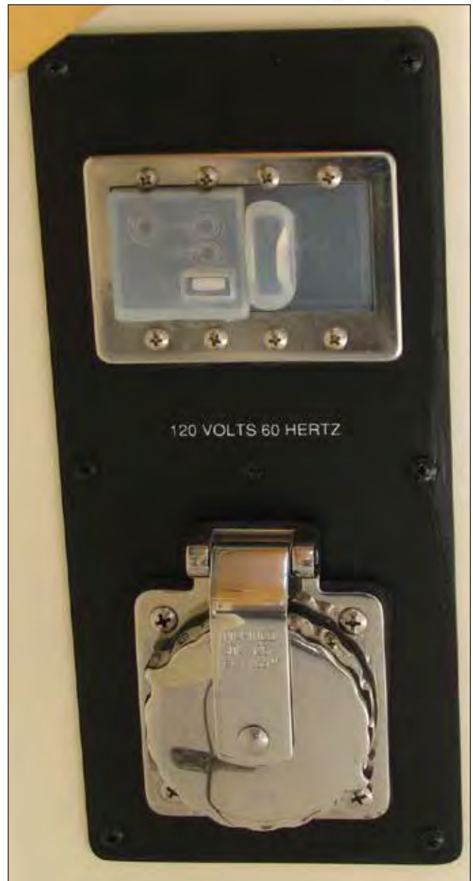
Boat AC Inlet, Main Circuit Breaker & ELCI
