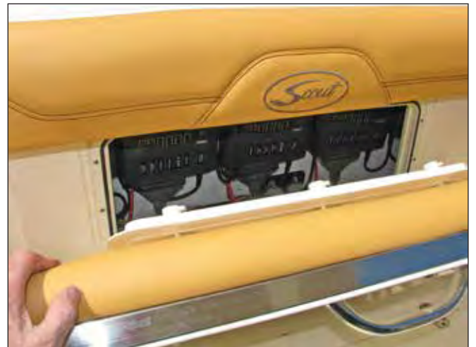
Aft Electrical Systems Compartment
