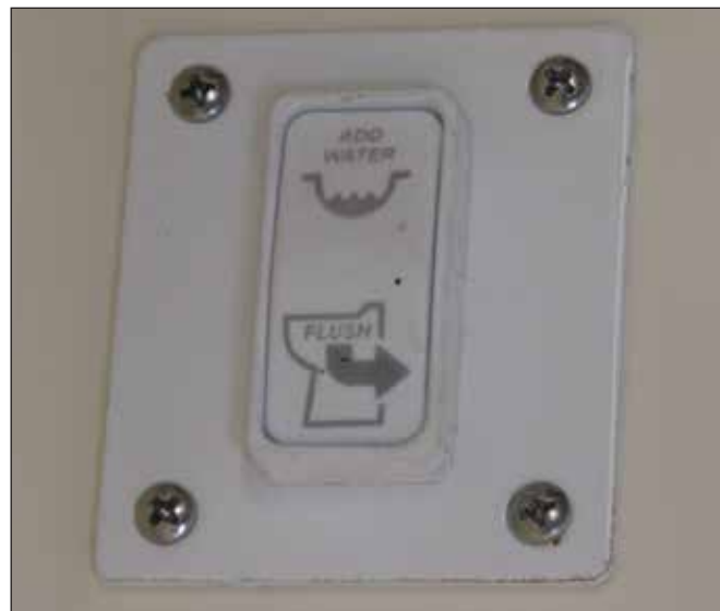
Marine Toilet Switch Panel
