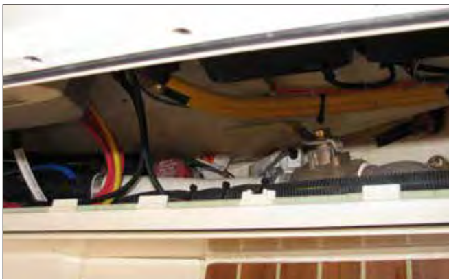
Forward Bilge Pump, Waste Discharge Pump & Overboard Valve
