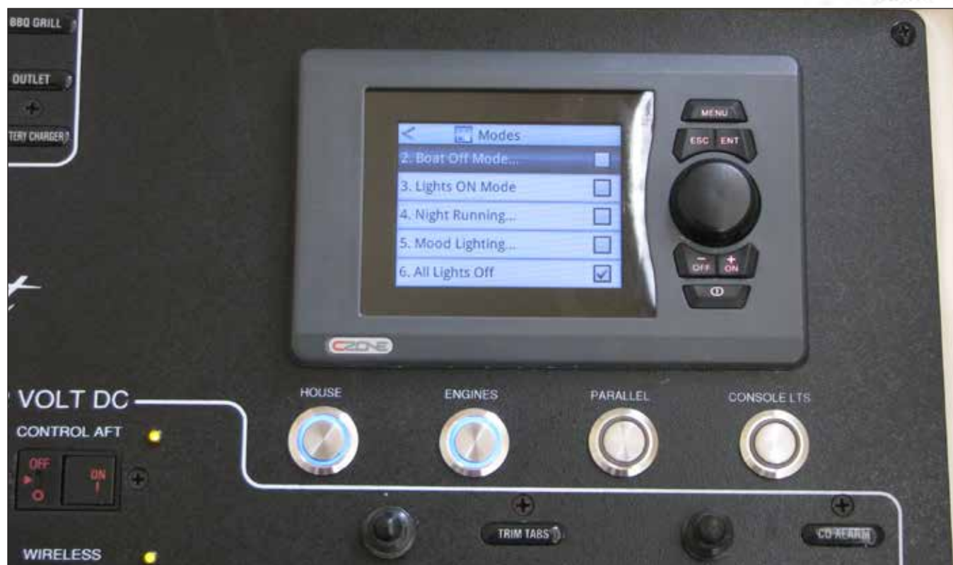
Battery & Parallel Remote Switches - House & Engine Battery Switches On CZone Control Panel
