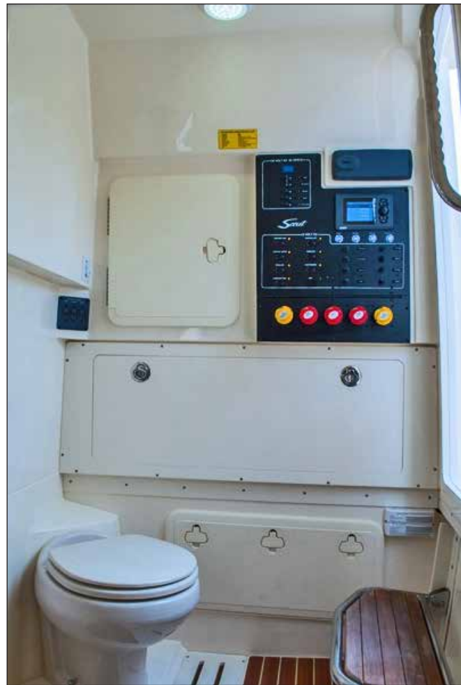
Equipment Access Doors
