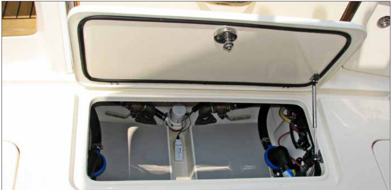
Aft Systems Compartment
