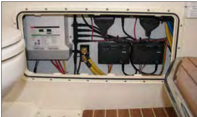
Forward Bilge Compartment, Battery Charger & Control Modules
