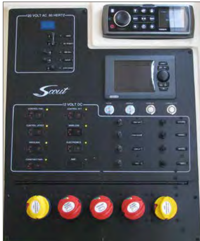
Cabin AC/DC Breaker Panel
