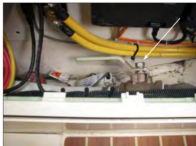
Forward Bilge Pump & Overboard Discharge Valve
