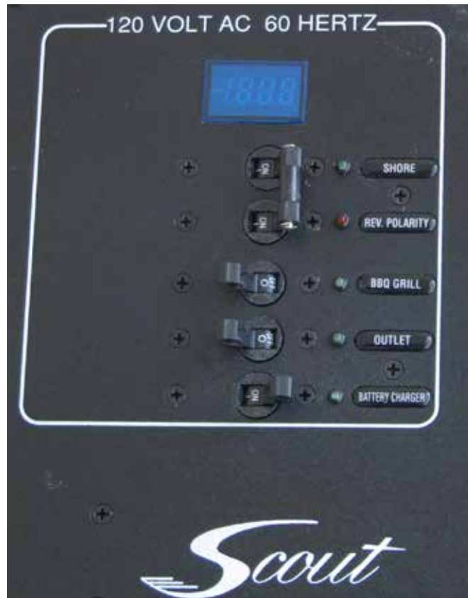
Cabin AC Panel Circuit Breakers & Reverse Polarity Light
