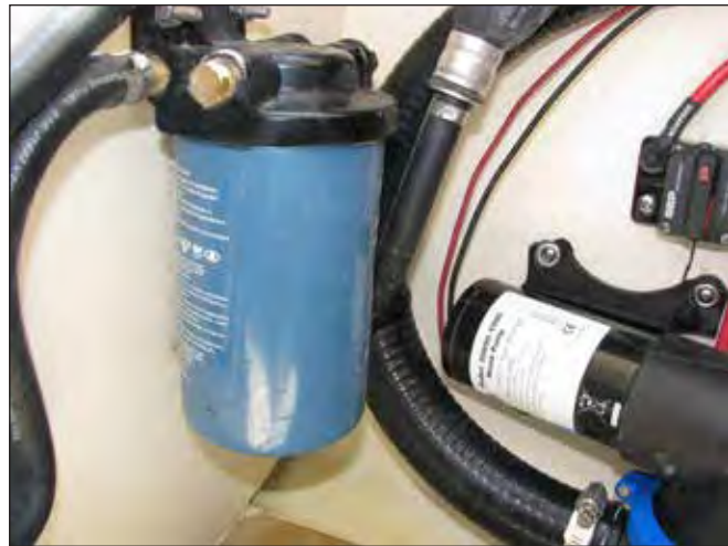
Engine Fuel Filter In Aft Systems Station
