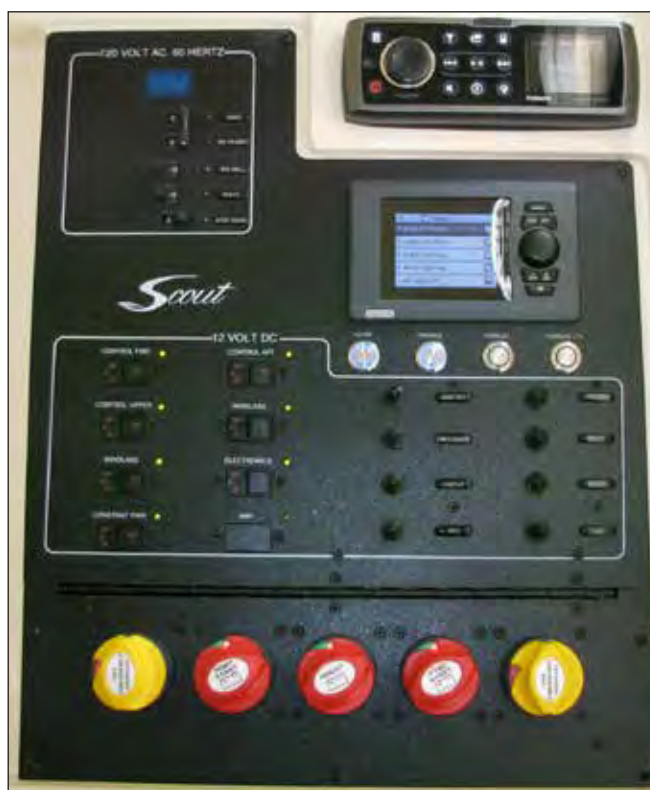
Battery & Parallel Switch Panel
