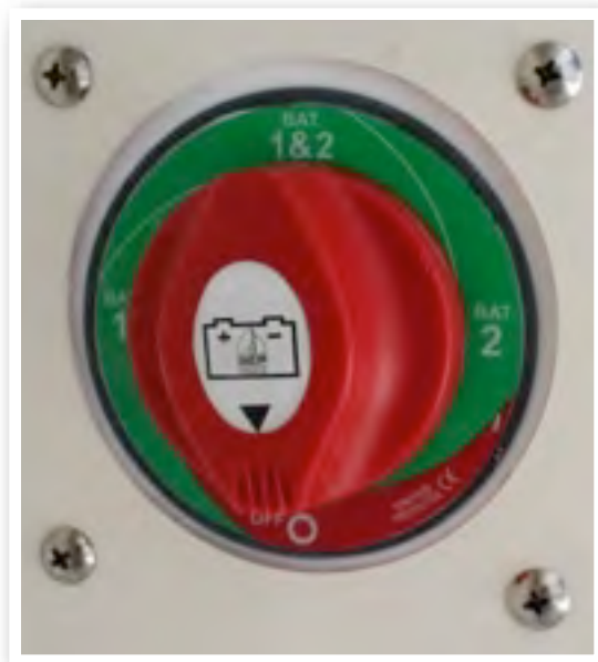
Battery Switch in the "off" Position
